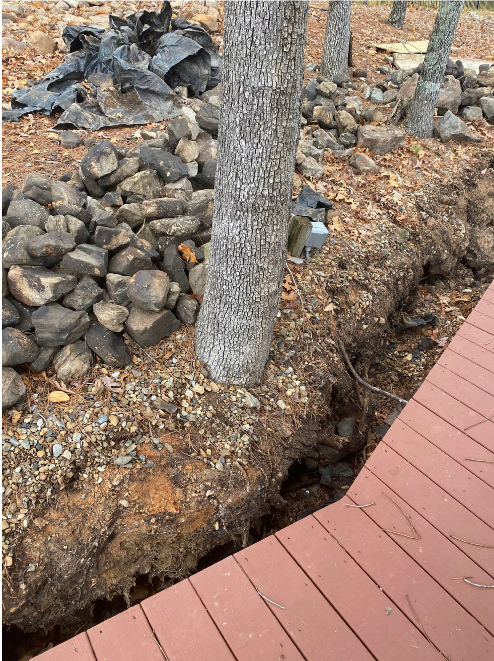
Figure 12: This erosion could not be seen until the riprap was removed. The void under the tree was deep enough that a full-size man could disappear under the tree. Thanks to the drawdown, it was caught, and tree removed before it fell on the roof of the dock.
