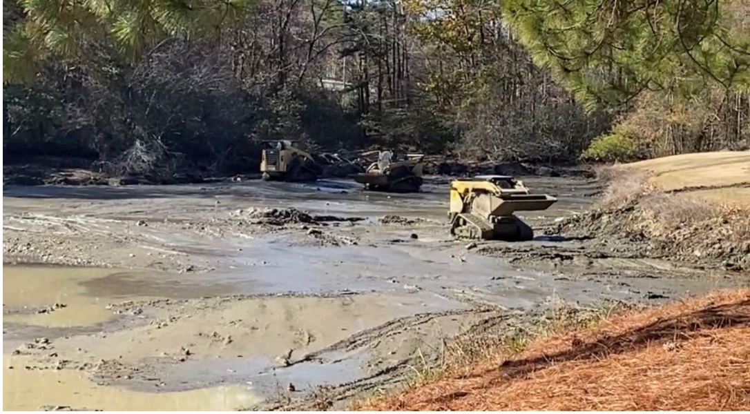
Figure 2 Three land operated dredging machines working diligently on the West end of Cortez Lake
