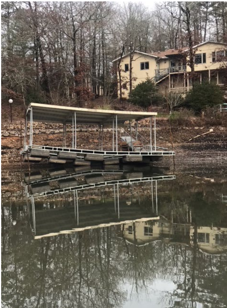
Figure 8: Dock is stuck on the guide pipes putting additional stress on the structure
