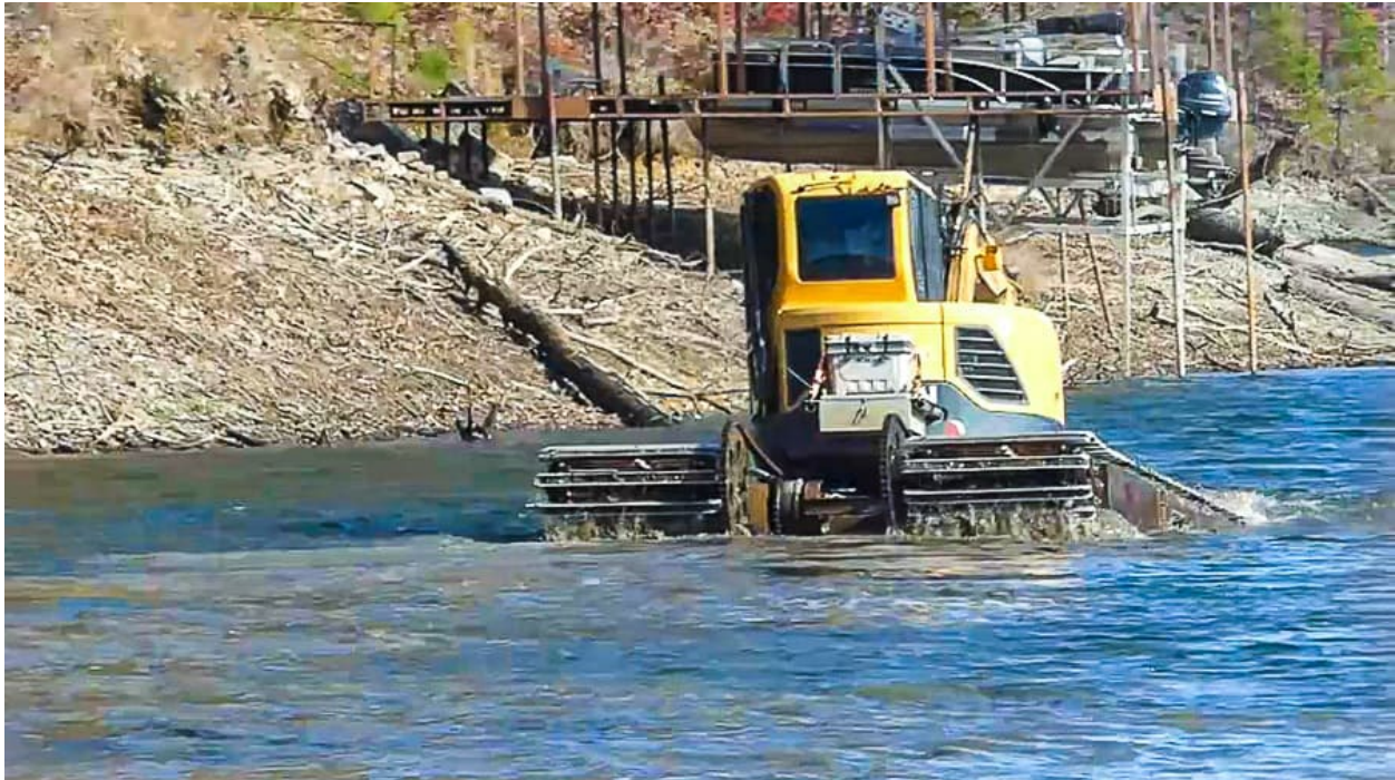
Figure 4: The amphibious dredging machine can work on land or water making it a very versatile alternative
