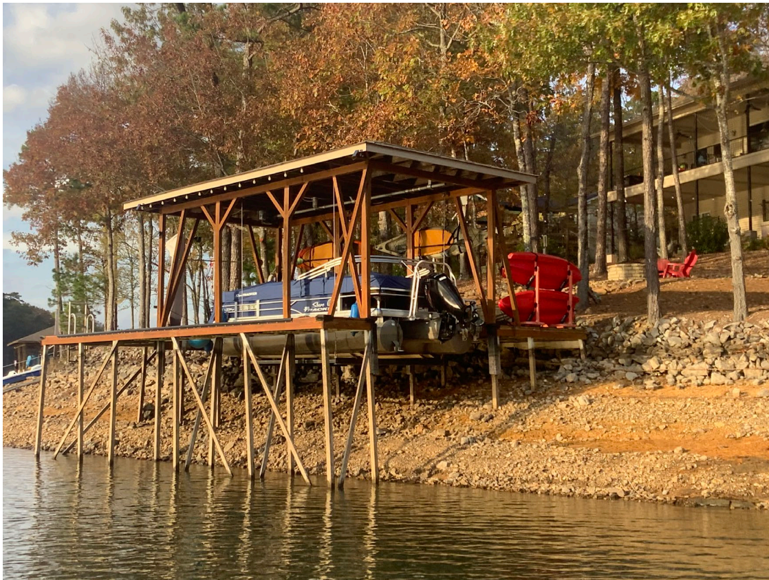
Figure 9: Fixed docks take away some of the concerns. You still must check your dock and shoreline.
