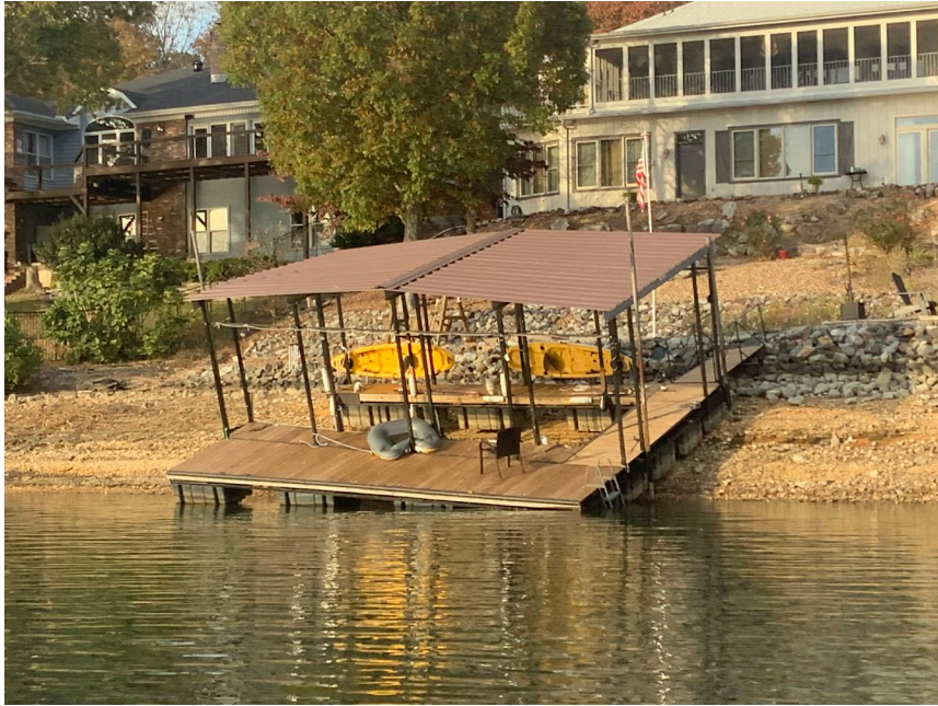
Figure 6: Dock is distorted and racked as it is hung up on a guide pipe
