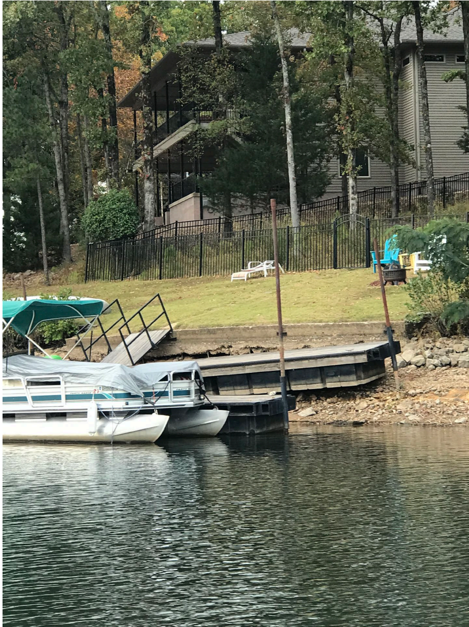
Figure 11: Notice the erosion under the base of the seawall. This was not noticeable at normal water level.
